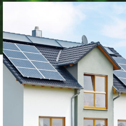
PHOTOVOLTAIC MODULES AND INVERTERS
